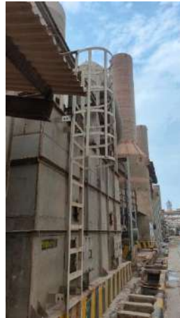
Gambar IX. 6 Stack/Tail Gas Scrubber Unit NPK Granulasi II
