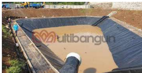
Gambar 6.5 Kolam Pengolahan Air Limbah (Sumber: https://multibangunpatria.com/proyek/kolam-pengolahan-air-limbah-pt-cakra-kencana-indah-salatiga/ )
