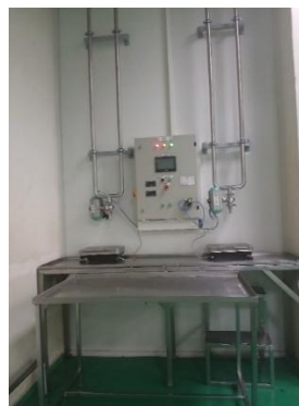
Gambar 22. Mesin Oil dispensing system
