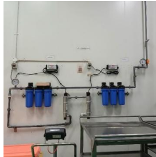
Gambar 23. Mesin Water dispensing system
