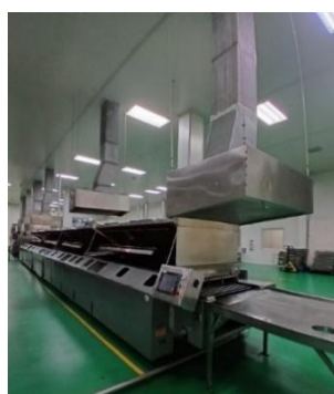
Gambar 18. Mesin Steam tunnel Panjang
