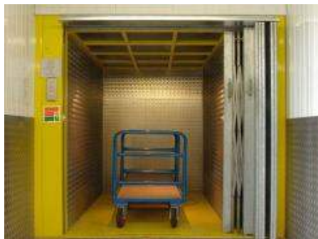
Gambar 5 49.Lift Barang & Disabilitas Sumber:arsitur.com
