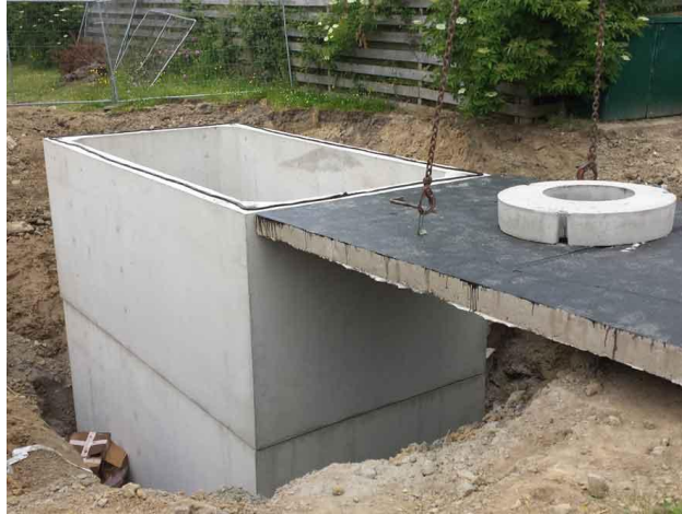
Gambar 2. 24 Reservoir Beton Cor (Sumber: https://aladintirta.blogspot.com )
