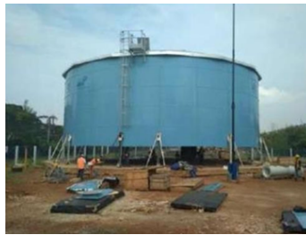
Gambar 2.13 Reservoir Tangki Baja
