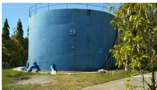
Gambar 2. 21 Reservoir Tanki Baja
