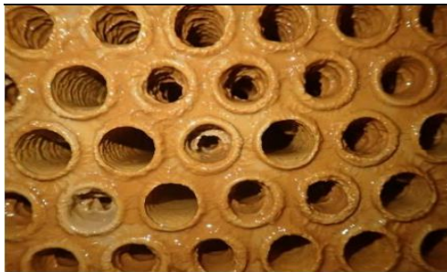
Gambar 1. Tube Brine Heater Sebelum Cleaning
