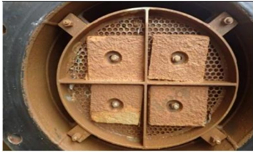
Gambar 7. Strainer Make Up Sebelum Cleaning
