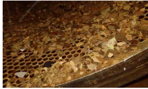
Gambar 8. Deposit Strainer Pompa Resirkulasi P1
