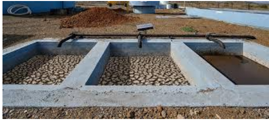
Gambar 2. 15 Bak Sludge Drying Bed
