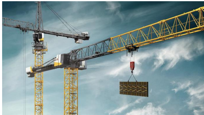
Gambar 3.1 Tower Crane Sumber: www.liebherr.com
