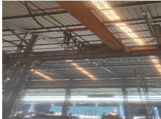
Gambar 3.4 Overhead Crane Single Girder
