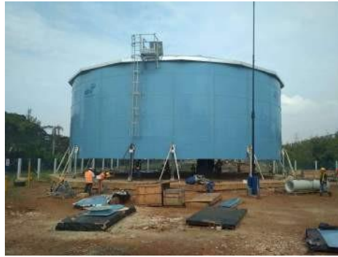
Gambar 2.10 Reservoir Tangki Baja
