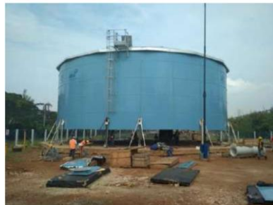
Gambar 2.25 Reservoir Tangki Baja
