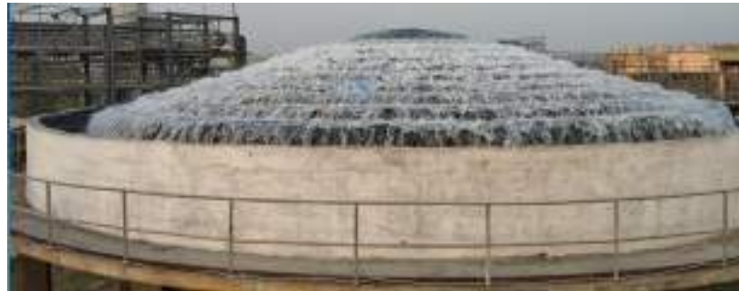
Gambar 2. 15 Multiple Platform Aerator
