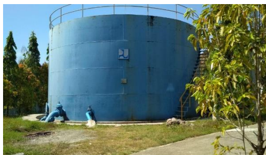
Gambar 2. 22 Reservoir Tanki Baja
