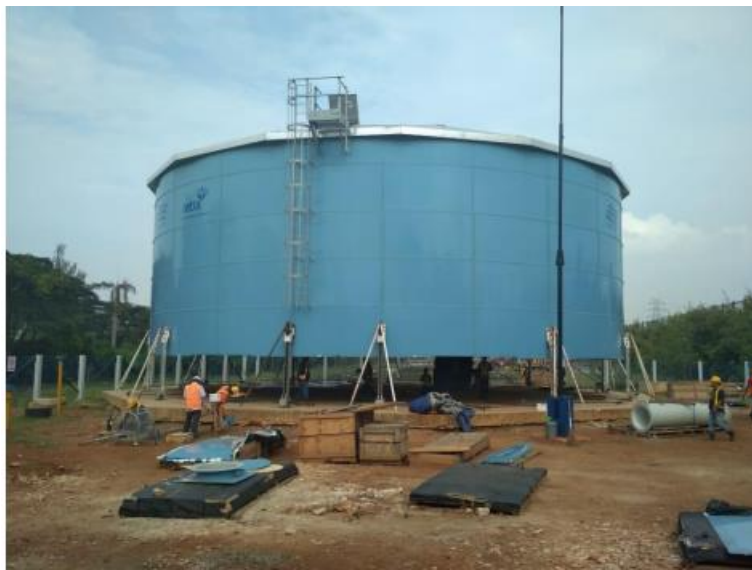
Gambar 2. 19 Reservoir Tangki Baja
