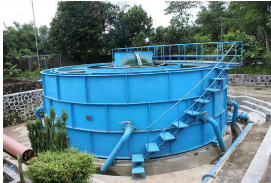
Gambar 2. 17 Reservoir Tangki Baja
