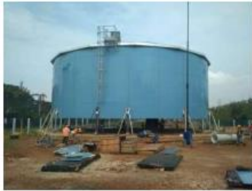
Gambar 2.10 Reservoir Tangki Baja
