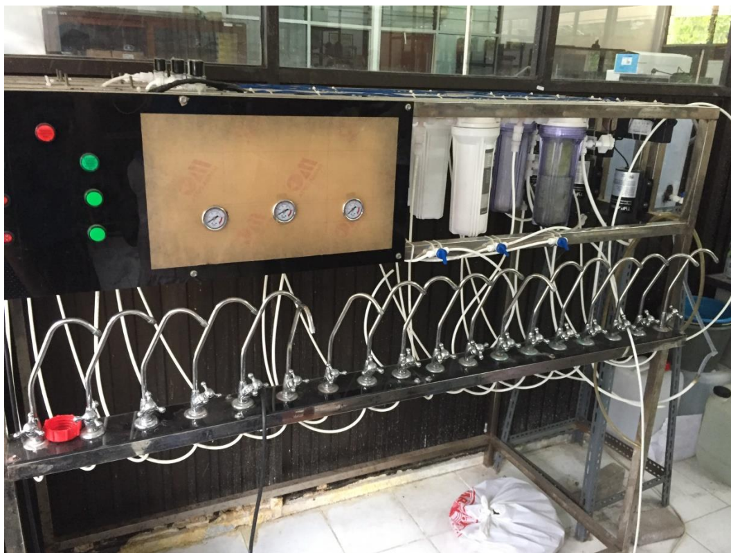
Rangkaian alat Reverse Osmosis
