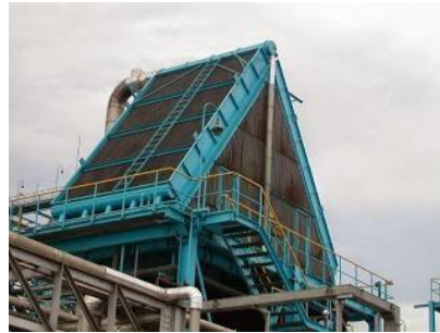
Gambar 2.4 Air Cooled Condenser
