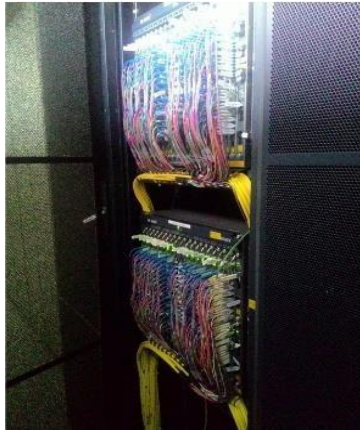
Gambar 3.1 Optical Line Terminal
