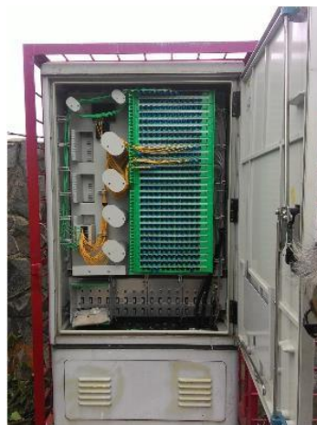
Gambar 3.4 Optical Distribution Cabinet
