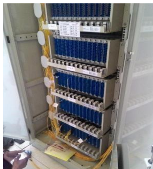
Gambar 3.2 Optical Distribution Frame
