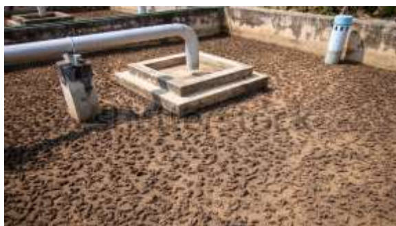
Gambar 2.16 Sludge Drying Bed
