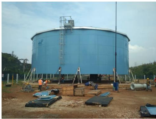
Gambar 2. 19 Reservoir Tangki Baja
