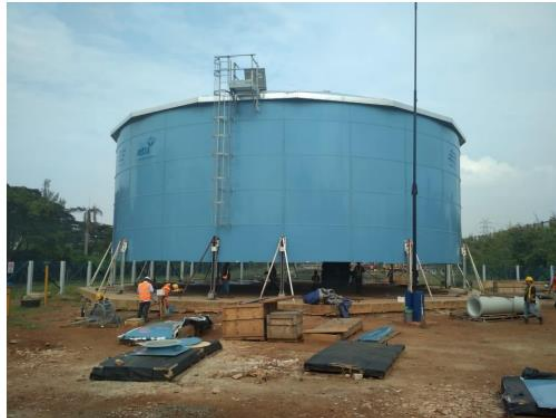
Gambar 2. 18 Reservoir tangki Baja
