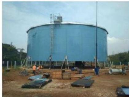
Gambar 2.16 Reservoir Tangki Baja
