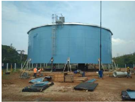
Gambar 2. 27 Reservoir Tangki Baja
