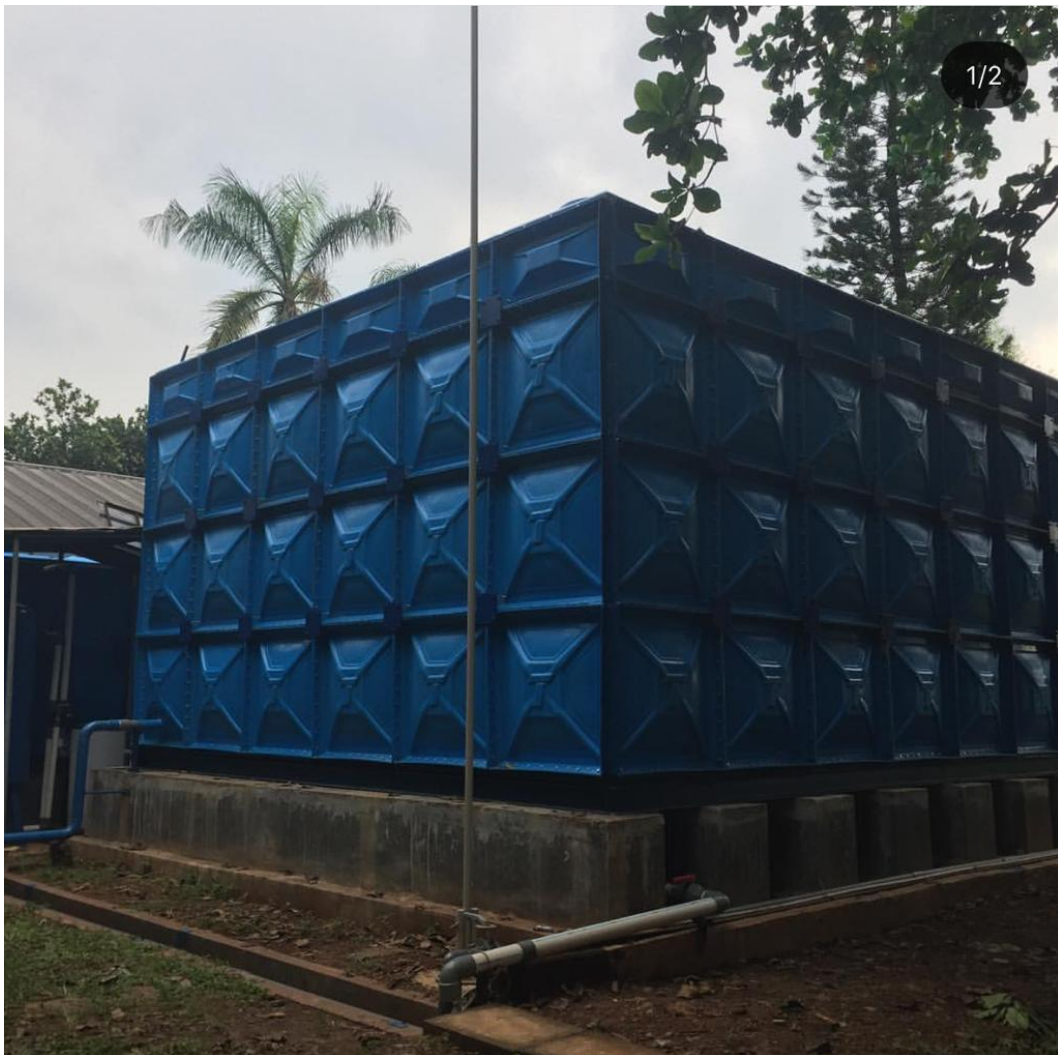
Gambar 2. 25 Reservoir Tanki Baja
