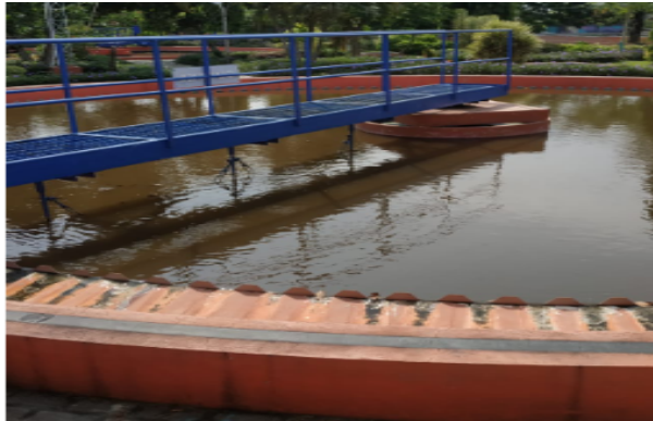
Gambar 2.9 Unit Final Clarifier
